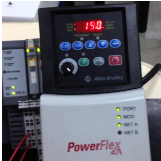
Figura 3.12 Inversor PowerFlex 40 de Allen Bradley.
