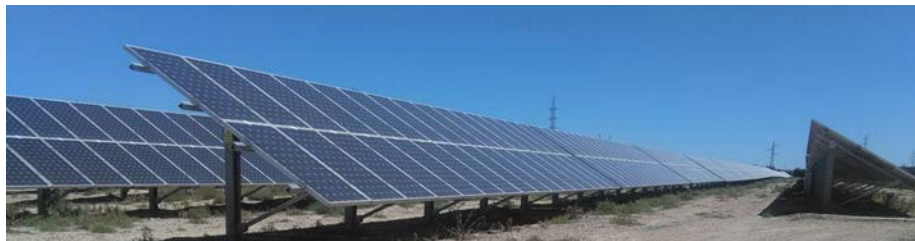
Figure 13: General view of the PV structures of the 3 MW PV plant analyzed.
