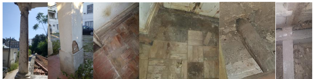
Figure 8. Set of photographs presenting anomalies verified in construction components [9].
