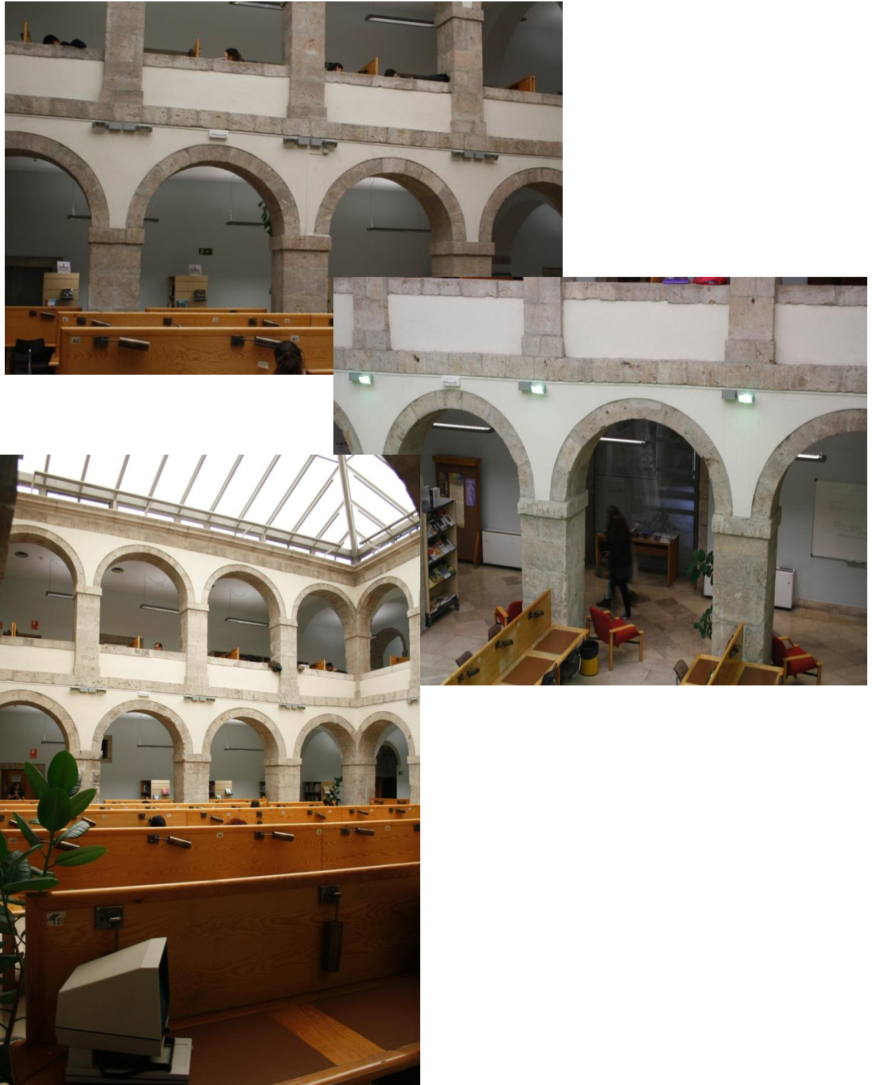
Figura 6.10. Luminarias sala central
