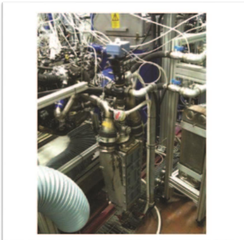
Figure 42. Compressed charge cooling system.
