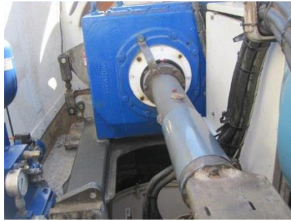
Figure 2.2.- Wind Turbine components into nacelle
