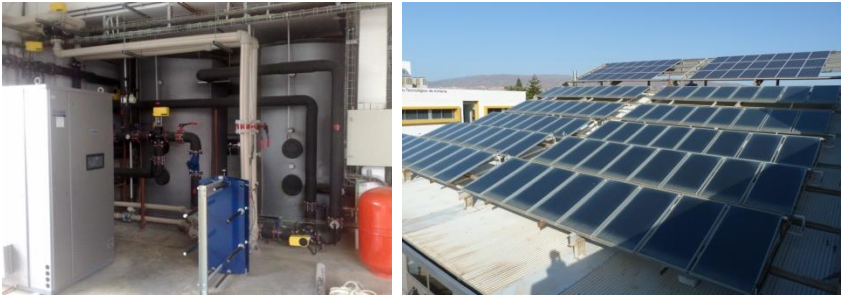
Figure 4.2.- Solar/gas heat supply system prototype built at Almeria
