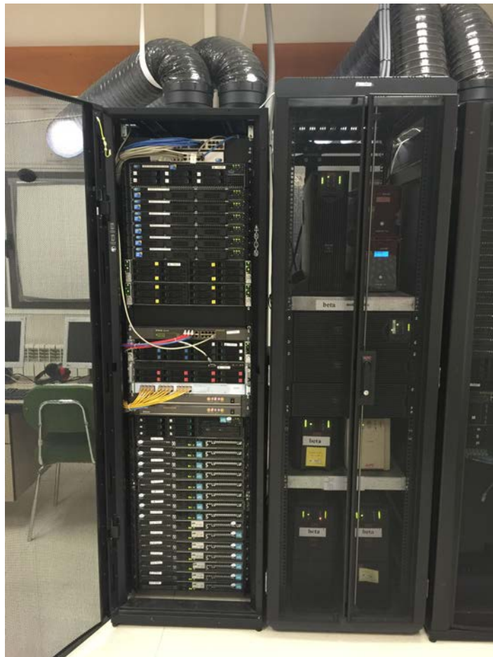
Figure 1.10: Picture of Beta and Gamma clusters and their UPSs taken in the Simulation Laboratory of the Higher Technical School of Telecommunications Engineering.
