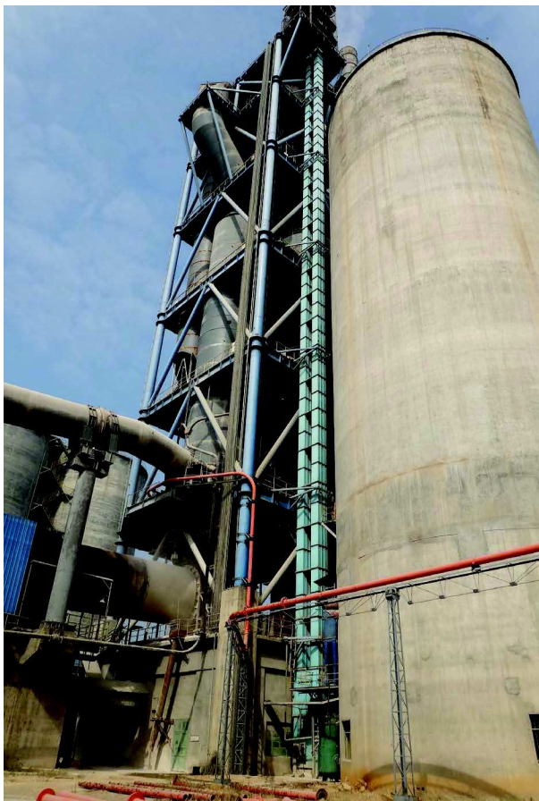
Sludge pipe at rotary kiln
