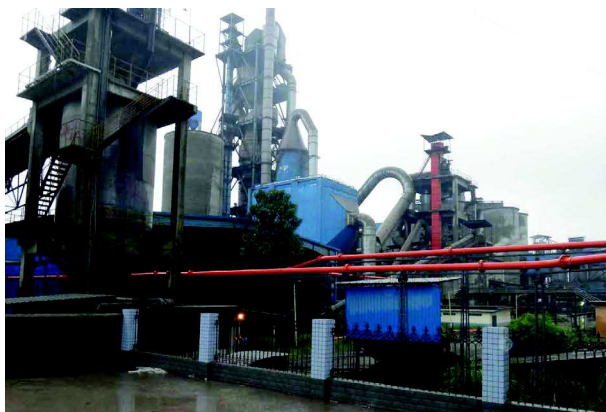
Sludge pipe routing
