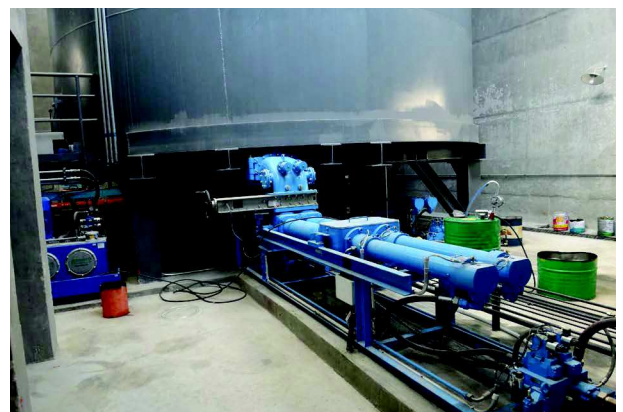
SH Pump installed under sludge reception silo
