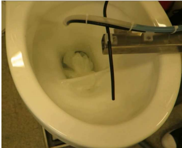
Figure 29 Toilet paper problem in Wostman toilet
