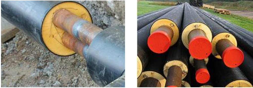
PICTURE 39. 2mpuk and Mpuk pipes of district heat network. (helsinginuuutiset.fi)
