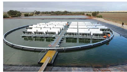
Figure 2.5: Jamestown Floating solar park.
