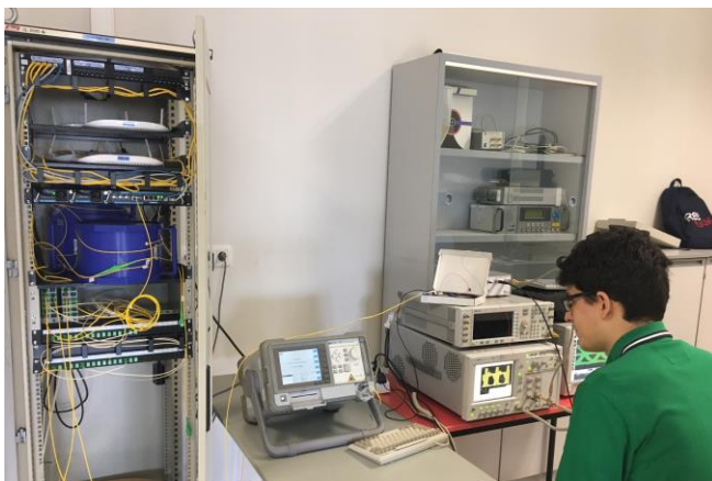
Figure 3. The GPON testbed and the optical instrumentation used in the optical communication laboratory
