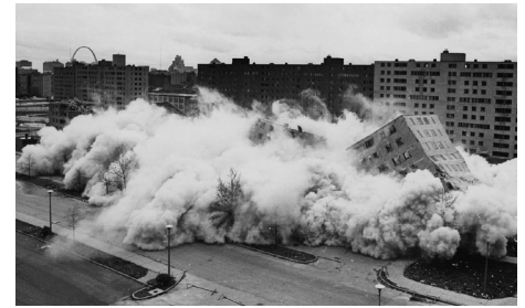
2 Demolición de uno de los bloques residenciales de Pruitt-Igoe, St. Louis (Missouri) 1972. [United States Department of Housing and Urban Development http://de.wikipedia.org/wiki/Pruitt-Igoe ]
