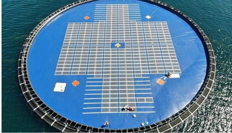
Figure 27. Swimming Solar Park by Statkraft, Albania
