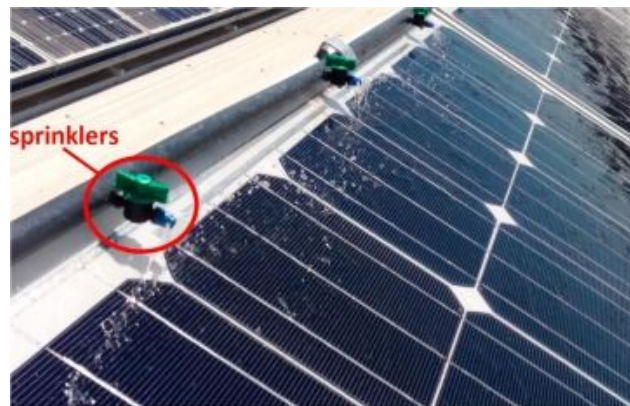
Figure 22. Visual of high- pressure sprinkler head for solar panel cooling system (Castanheira A., Fernandes J., Branco C., 2018)
