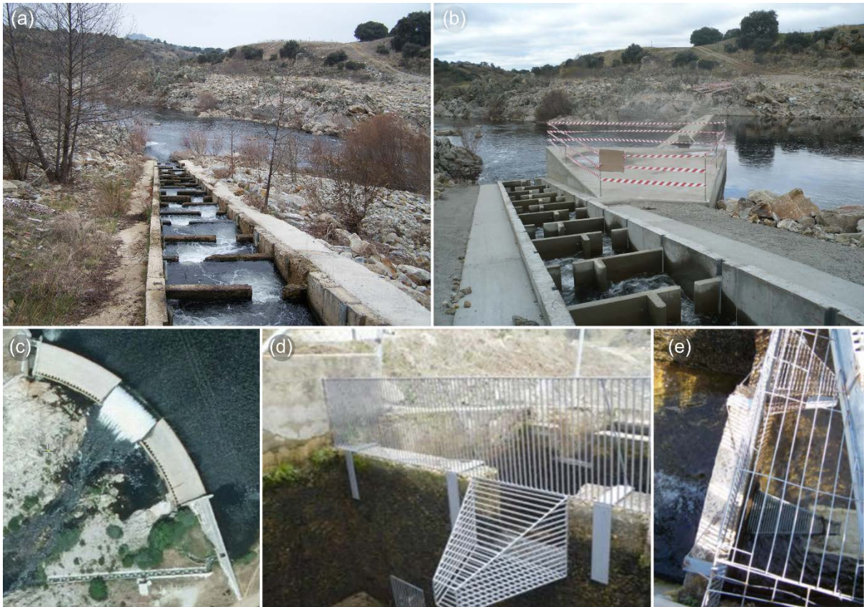
Figure 11. Tormes River: (a) old fishway (2012–2013); (b) retrofitted fishway and small attraction weir (2014–2016); (c) plant view of the dam and old fishway; (d) capture pool with funnel only in the notch; (e) funnel in both notch and orifice. Source: GEA-Ecohidráulica.
