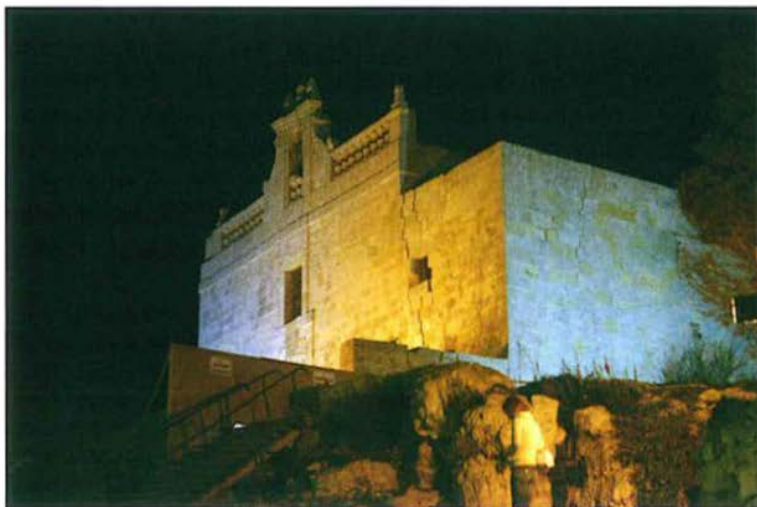
Plate 2: The chapel dedicated to the Our Lady of Annunciation, lit up during the Holy Week, visible damage and cracks could be clearly seen
