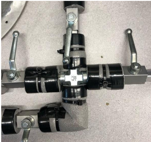
Figure 73 Insulation for pipes
