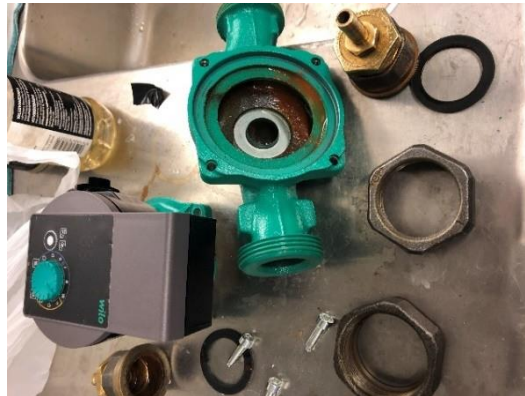
Figure 34 Corrosion on new pump
