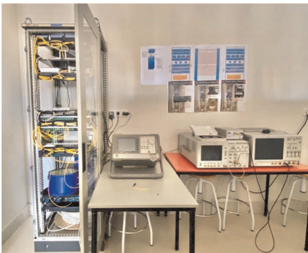
FIGURE 9 The GPON (passive optical networks based on the Gigabit standard) testbed and the optical instrumentation used during the experimental sessions
