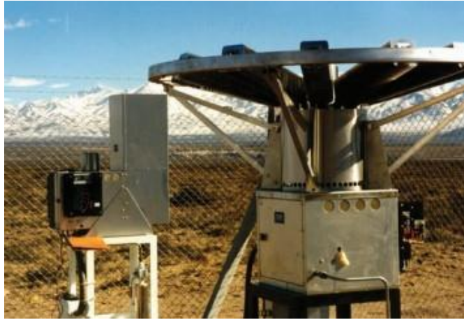
Figure 36. 550 W TEG installation in Argentina [36]
