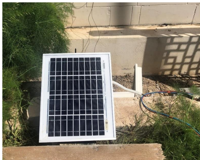
Figure 39. Solar panel that powers the datalogger's battery
