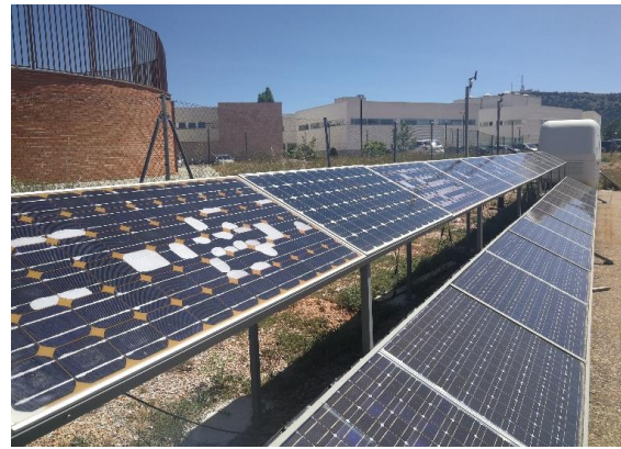
Figure 3: PV field of the Campus Duques de Soria, University of Valladolid.
