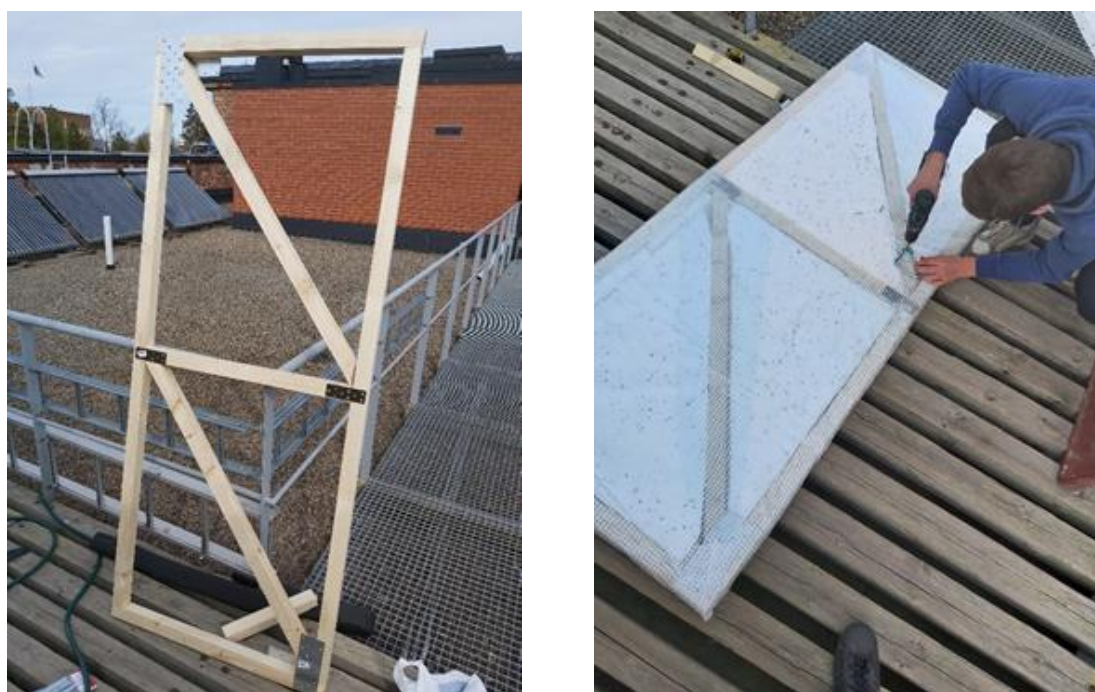
Figure 80. Construction of the door. Frame on the left and almost end product on the right.
