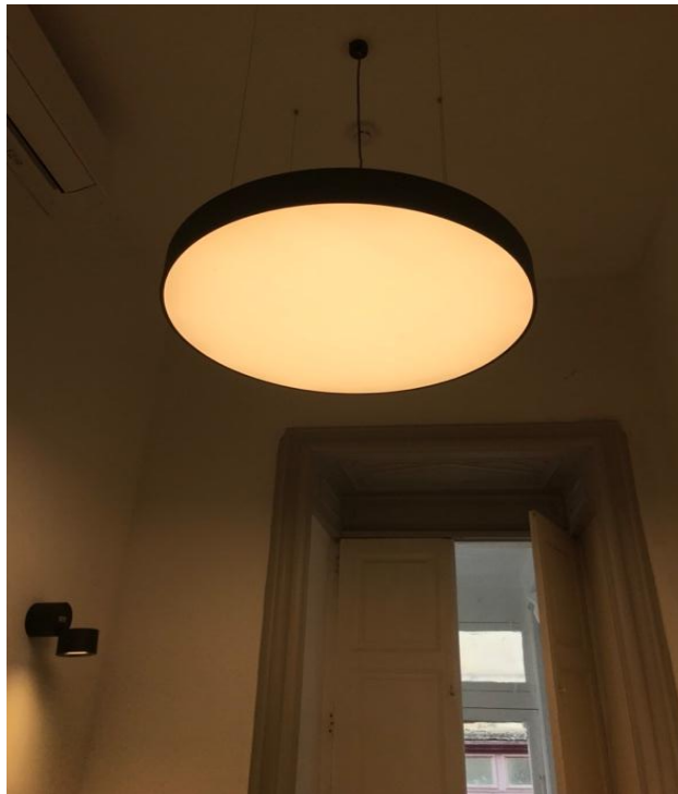
Figure 53. Large lamp in an office of small dimension
