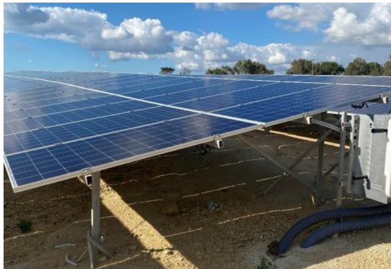
Figure 35. Inclination and orientation of PV modules in PV Farm 2.
