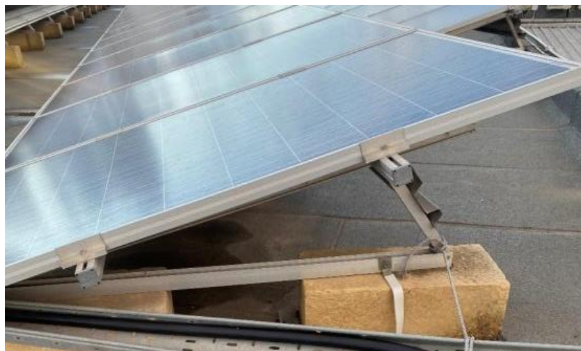
Figure 39. Inclination of first type of PV modules in first roof of PV Farm 3.
