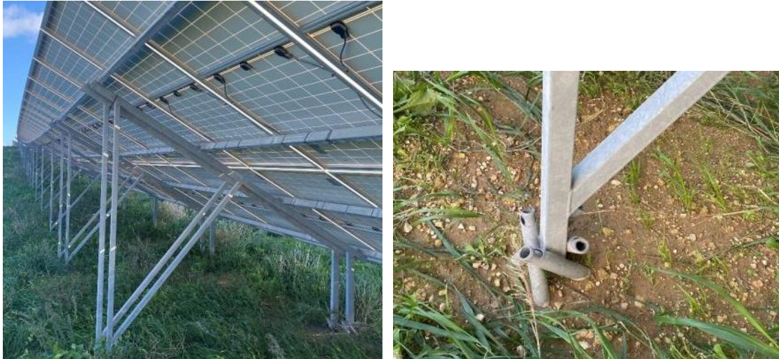
Figure 31. Back part of the PV modules and anchoring to the ground in PV Farm 1.
