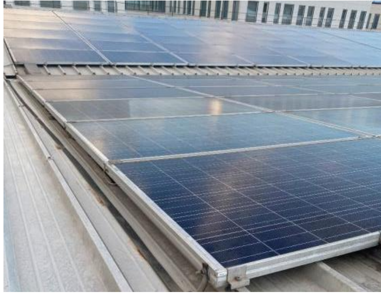
Figure 40. Inclination second type of PV modules in first roof of PV Farm 3.
