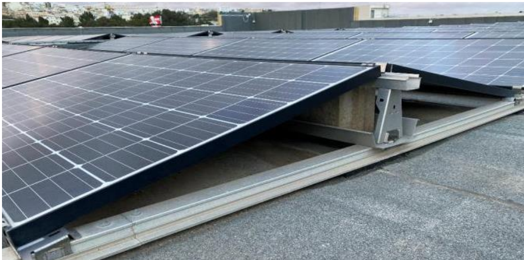
Figure 41. Inclination of PV modules in second roof of PV Farm 3.
