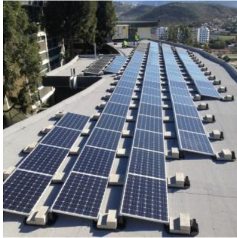
Figure 2. PV rooftop installation with ballasted mounts [14].
