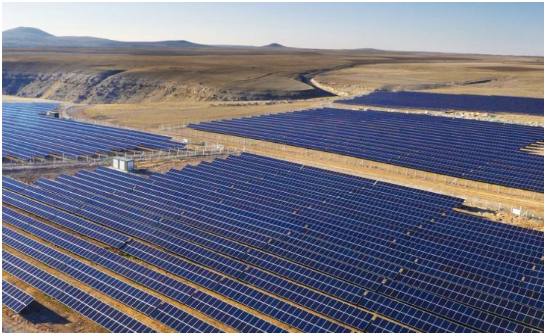
Figure 17. Ground mount PV installation with tilted angle [47].
