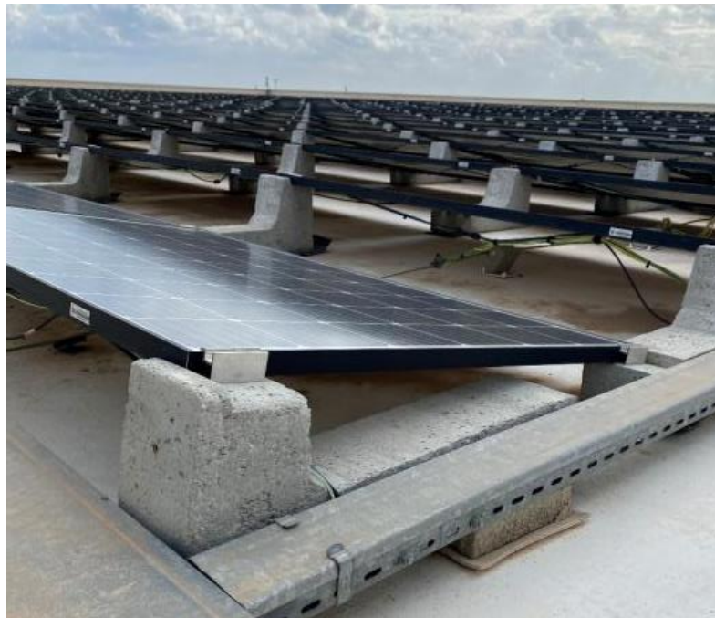
Figure 47. Inclination and orientation of PV modules in PV Farm 4.
