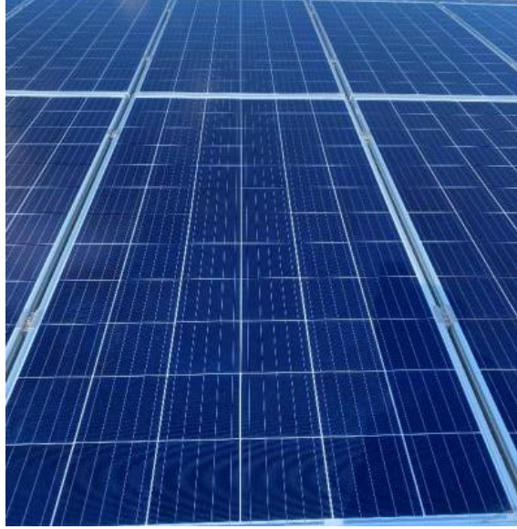
Figure 34. Solar module of PV Farm 2.
