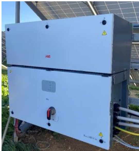
Figure 32. String solar Inverter PVS-175-TL at PV Farm 1.
