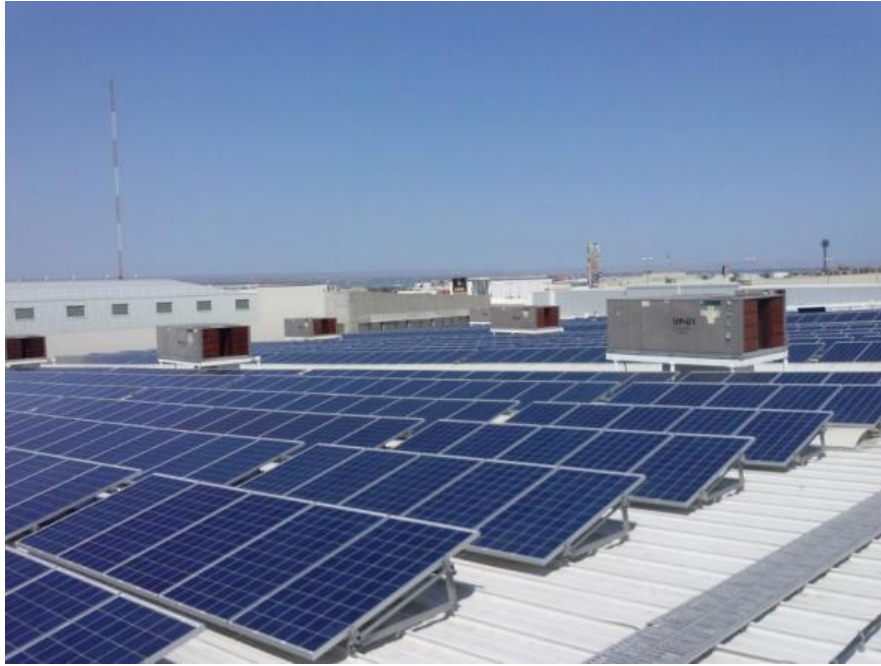
Figure 16. Rooftop PV installation with a tilted angle [47].
