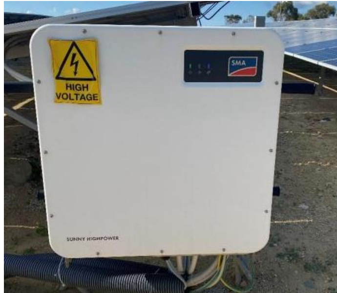
Figure 37. String solar inverter Sunny Highpower 150-20 in PV Farm 2.
