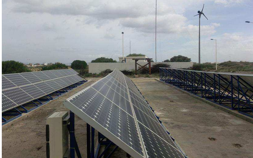
Figure 3.11: Power energy system for the RO pilot plant: Solar panels and wind turbine.
