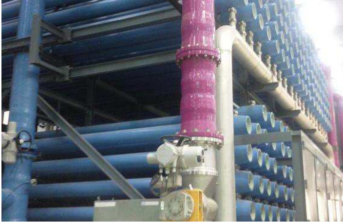
Figure 1.12: Racks of RO pressure vessels. Desalination plant of Barcelona-Llobregat (Spain), property of the company ATLL.
