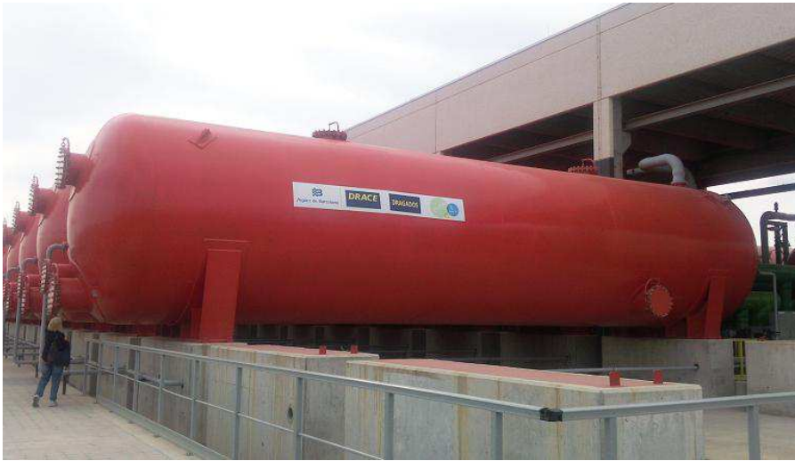
Figure 1.17: Pressurized sand filters. Desalination plant of Barcelona-Llobregat (Spain), property of the company ATLL.
