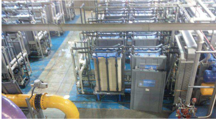
Figure 1.7: EDR system. Water purification plant of Abrera (Spain), property of the company ATLL.
