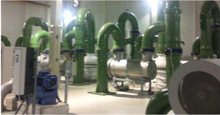
Figure 1.19: Ultraviolet disinfection chambers. Water purification plant of Sant Joan Despí (Spain), property of the company Agbar.
