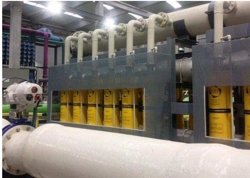
Figure 1.21: Rack of pressure exchangers, from the company ERI (type PX). Desalination plant of Barcelona-Llobregat (Spain), property of the company ATLL.
