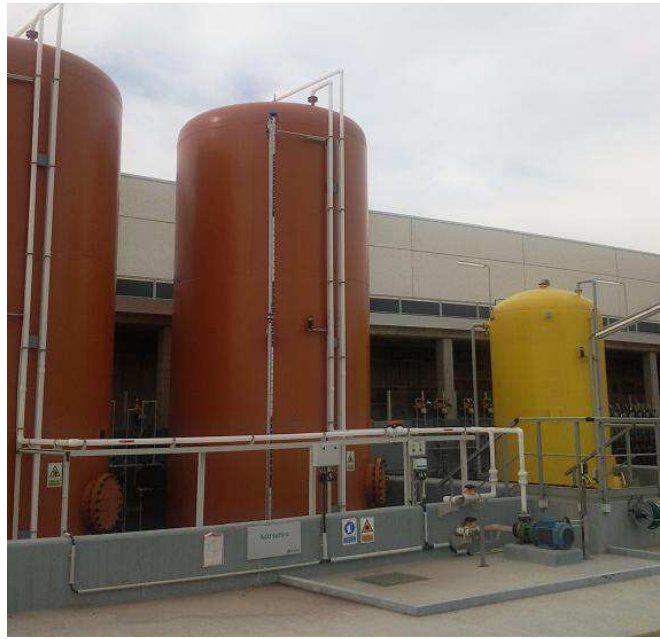
Figure 1.16: Tanks for the addition of chemicals. Desalination plant of Barcelona-Llobregat (Spain), property of the company ATLL.
