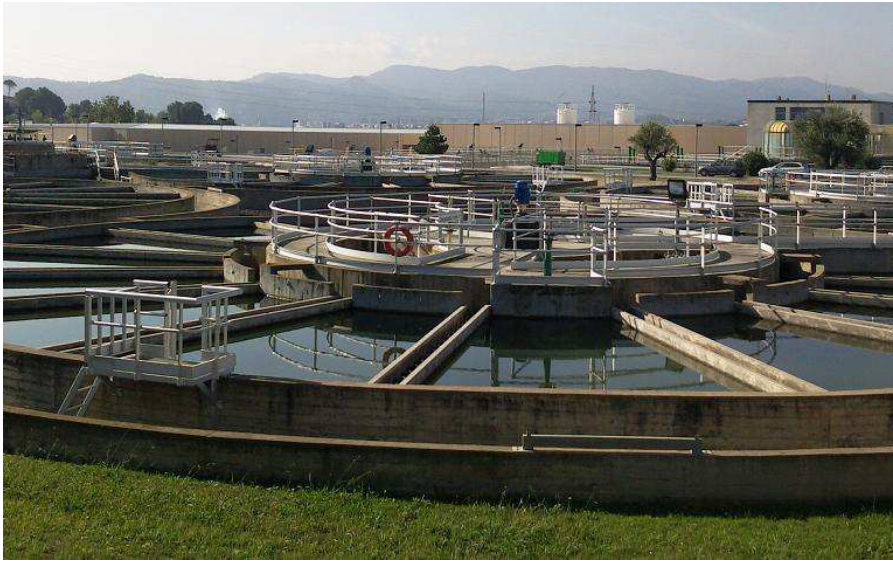
Figure 1.15: Decantation tanks. Water purification plant of Abrera (Spain), property of the company ATLL.
