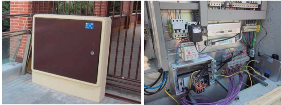
Figure 8: Measurement system installed in the electrical cabinet.
