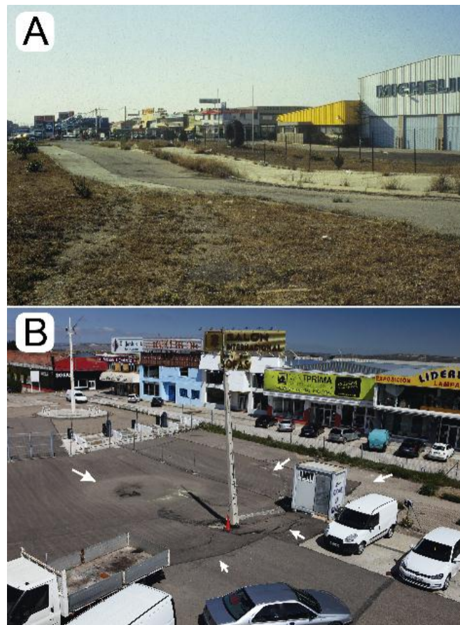
Figure 5. Images of the Logroño highway sinkholes. (A) Photograph taken on June 1996 at the NE sector of sinkhole 1 before the enlargement of the highway and the construction of the currently existing department store. Note the conspicuous sagging of the service road and the sidewalk. (B) Image of sinkhole 2 taken on April 2016 affecting a recently asphalted surface within a fenced area. The left arrow points to the deeper part of sinkhole and the arrows on the right mark the outermost cracks.
