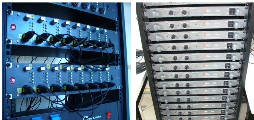
Figure 9. Preamplifiers and amplifiers.
