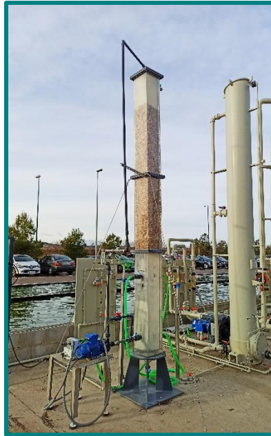
Figure 8.3. Siloxanes removal unit: pilot scale two-phase partitioning biotrickling filter.
