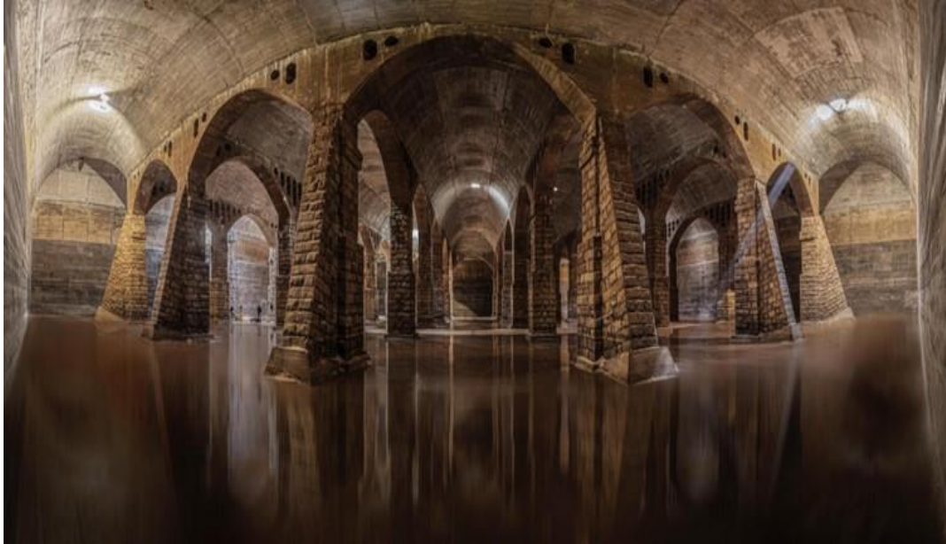
Figure 16: Luqa Reservoir; known as the 'sunken cathedral', constructed at around 1907. Courtesy of the Malta Water Services Corporation.
