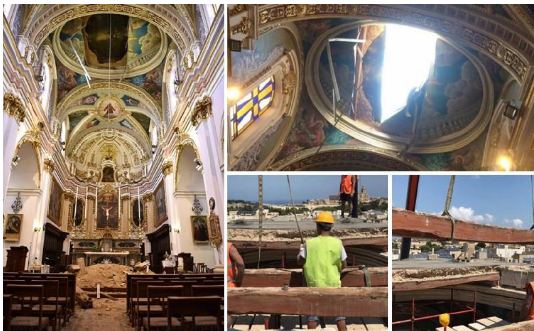
Figure 9: Church of Our Lady of Jesus (Ta' Giezu), Rabat, Malta. 16th Century Church Ceiling Collapse on 23 August 2017. Pictures courtesy of the Franciscan Fathers.
