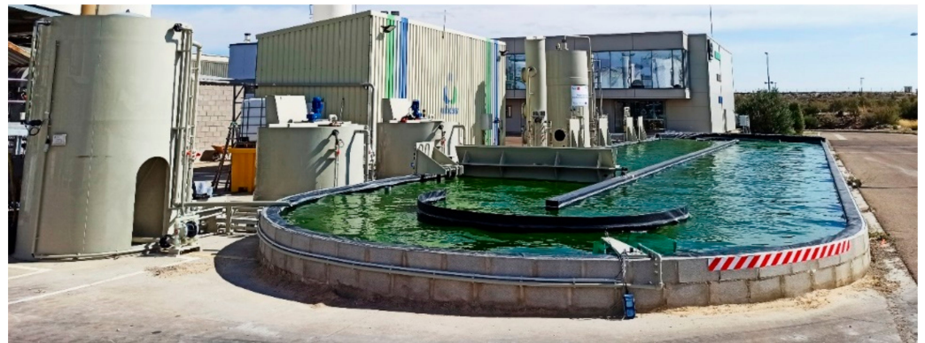
Figure 15. Photosynthetic biogas upgrading plant under validation in URBIOFIN project.
