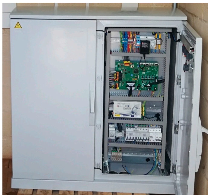
Figure 4. Bidirectional power inverter of the Campus Duques de Soria of the University of Valladolid.
