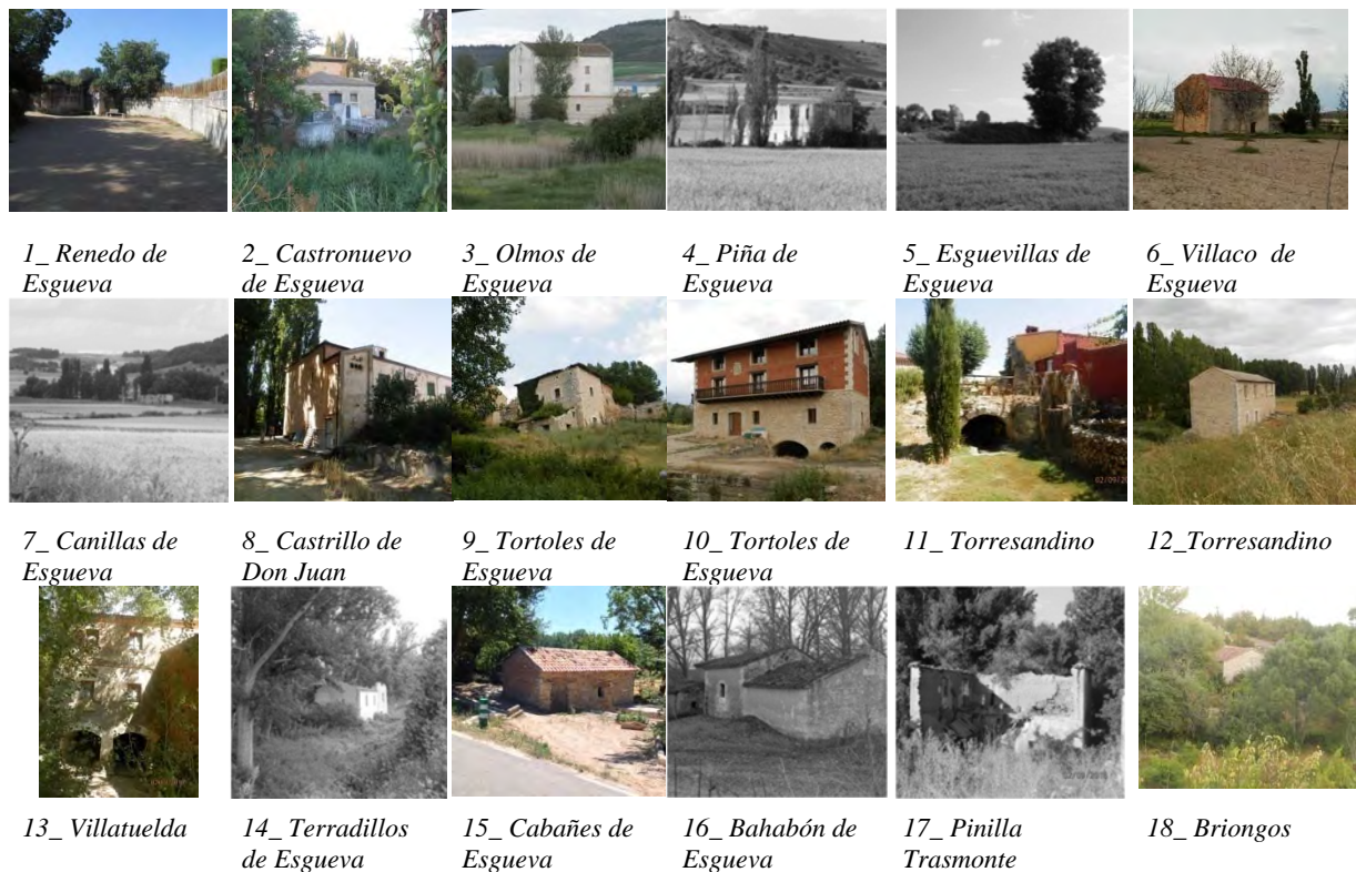
Fig. 3 –Current status of the mills located along the entire course of the River Esgueva. Reading of images according to the sense of the course: from left to right and from top to bottom. Black and white mills in danger of disappearing by their state. Author source AEG. – Source: photo of the authors
