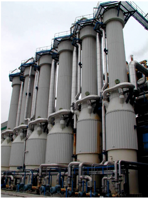
Fig. 2. Six evaporation units for the evaporation section in a beet sugar factory in Spain.
