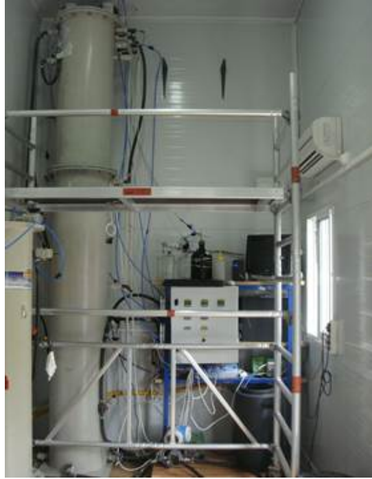
Figure 3.8. AnSMBR pilot plant: UASB reactor with polymeric hollow fiber membrane submerged internally on top.
