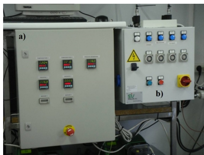
Figure 3.5. Electric panels of the pilot plant: a) BS2100 regulator, b) timers OMRON.
