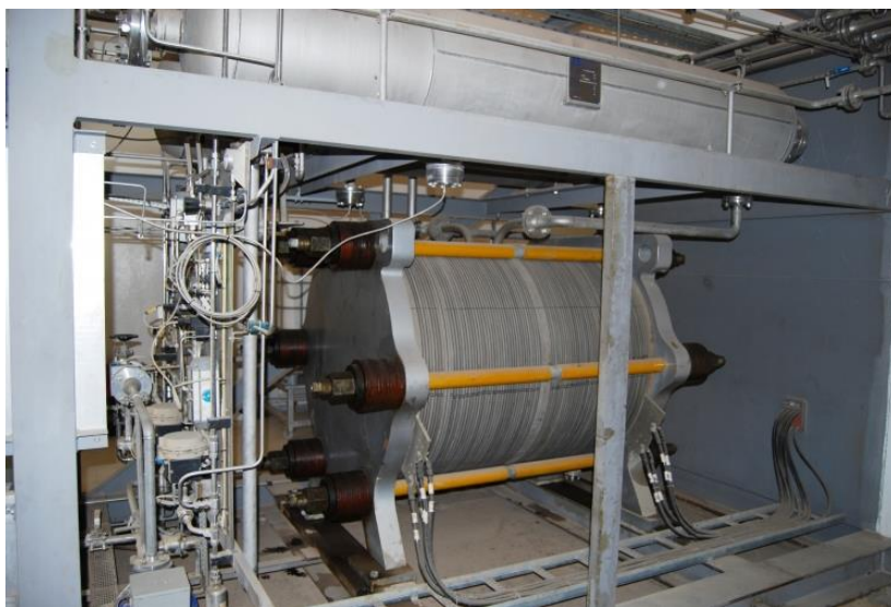
Figure 2.20-Alkaline electrolyzer stack filled with a KOH pure solution ( http://www.alnooroils.com/en/post.php?id=26 ).
