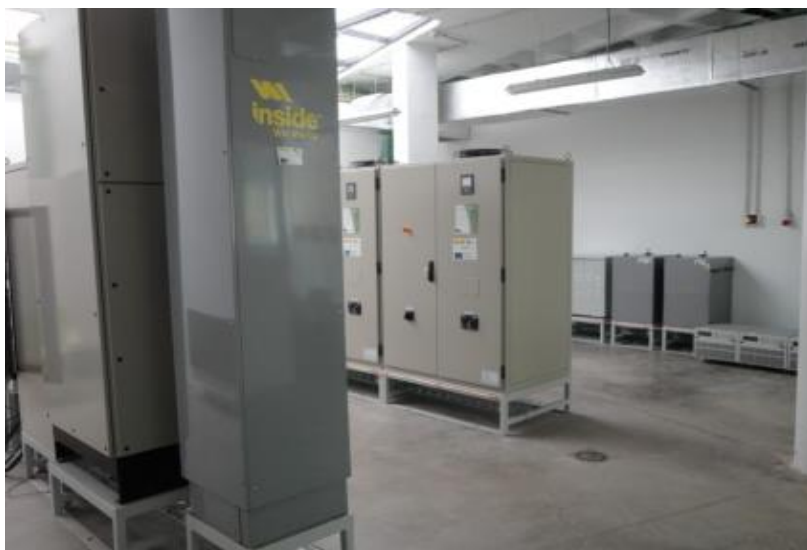
Figure 5.7 – Battery and ultracapacitor in the CNH2 ( http://cnh2.es/docs/tripticos/IV.%20Triptico_Lab.Microrredes_CNH2.pdf )
