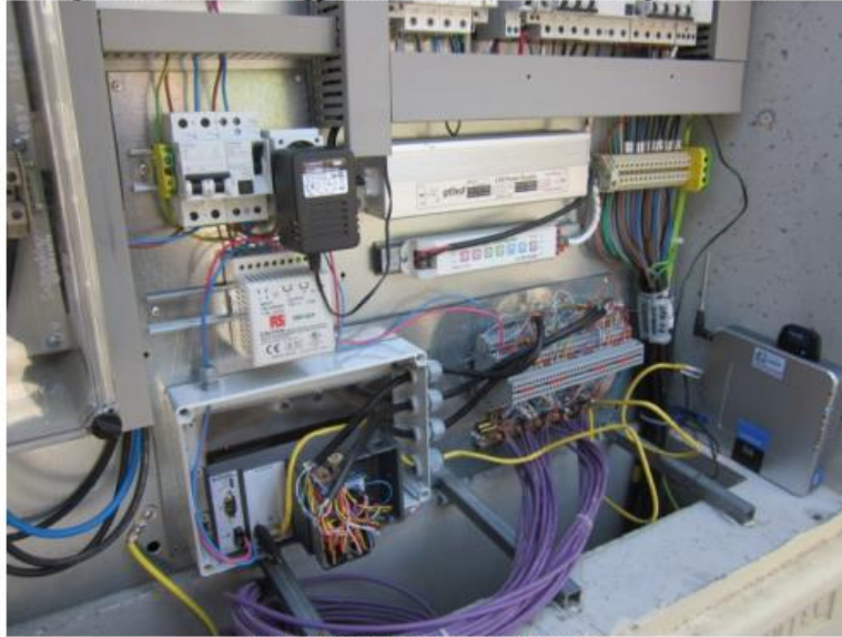
Figure 4. Data logger, router and other devices.
