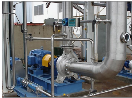
Circulation system of the finisher
