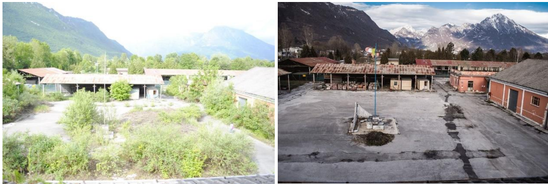
Fig. 58 and 59: the Piave barracks in summer 2013 (on the left) and in winter 2018 (on the right).
