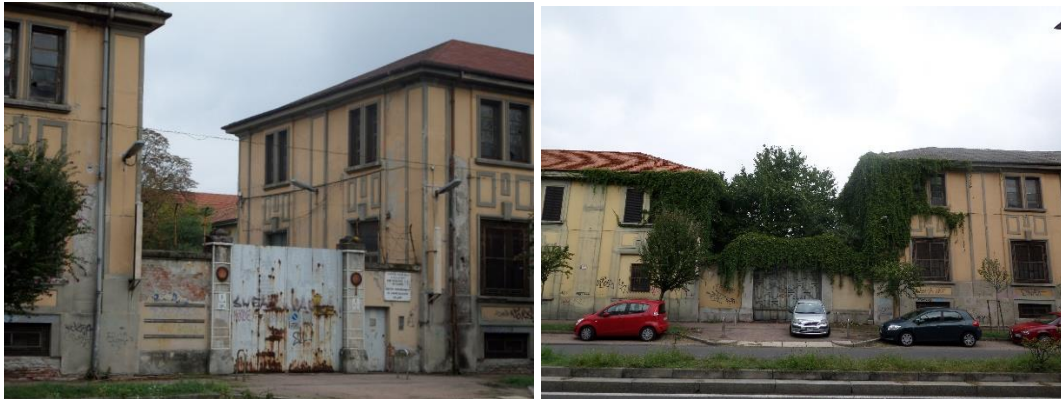
Fig. 49 and 50: images of the state of abandonment and degradation of the Baggio warehouses.
