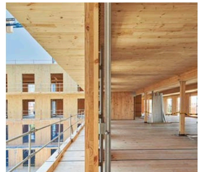
CLT panels in floors and walls and glulam beams and columns. Eaoin https://n9.cl/a4o21
