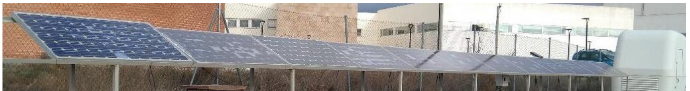
Figure 1. Experimental installation implemented in the Duques de Soria University Campus of the University of Valladolid, Soria (Spain).
