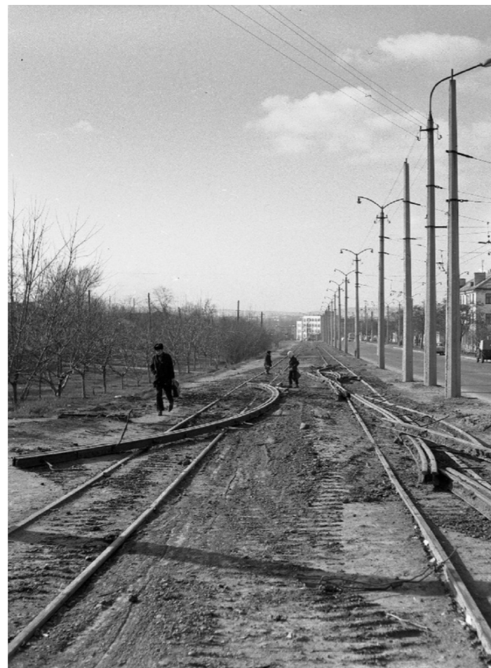
Fig. 79. The dismantling of tram lines on Pobeda Avenue in 1971. Source: GUP RK Krymtrolebus, www.transphoto.org .
