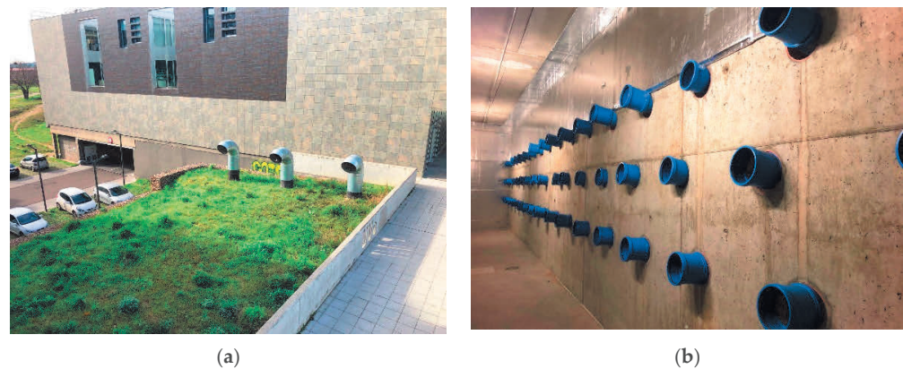
Figure 1. Earth-to-air heat exchanger at the LUCIA building: (a) outside; (b) inside.
